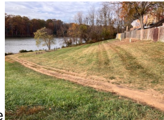
Current deteriorating hillside
